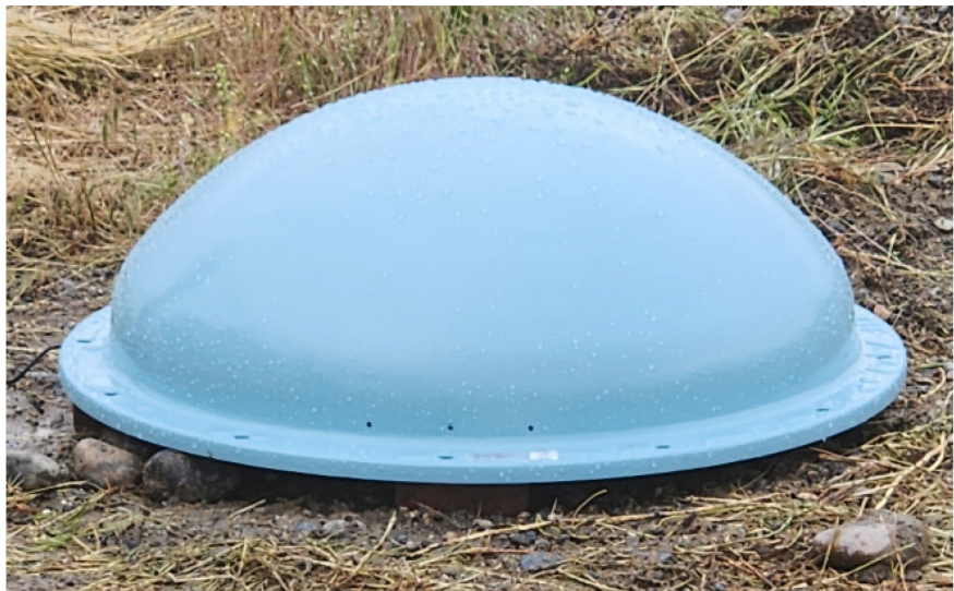
Figure 2. The fiberglass hemispherical radome is leveled and centered over the GPS antenna [1].
