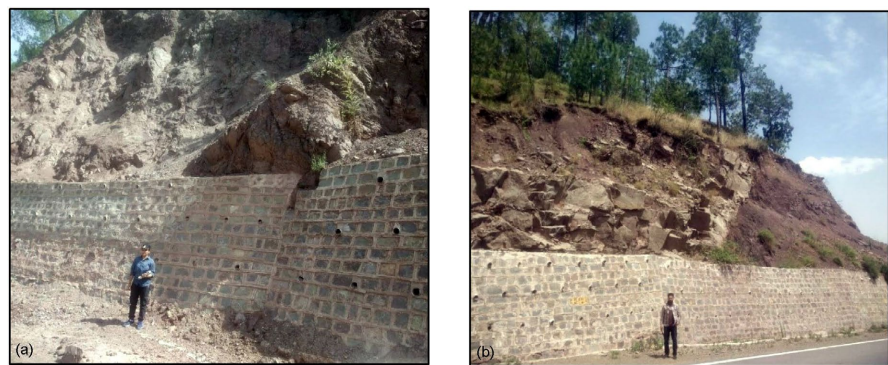
Figure 2. Field images of landslide features in the research region. (a) A small scale landslide with a visible escarpment indicating slope failure; (b) Rock mass instability with displaced boulders and imbalanced rock formations.
