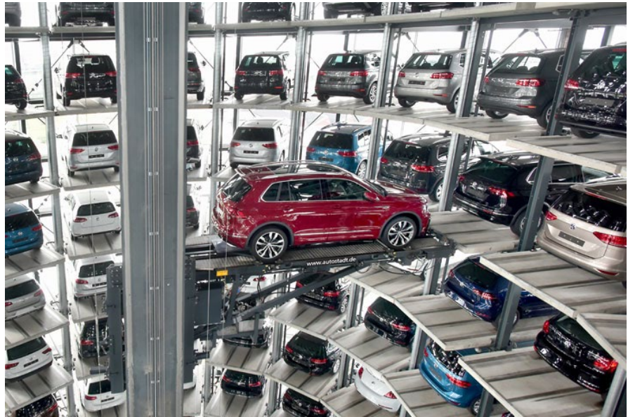
Figure 12. Automated car lift parking systems: (Used with permission) ( https://blog.getmyparking.com/2017/08/30/an-overview-of-automated-parking-system-and-its-types/ ) [Site visited 07/06/26].
