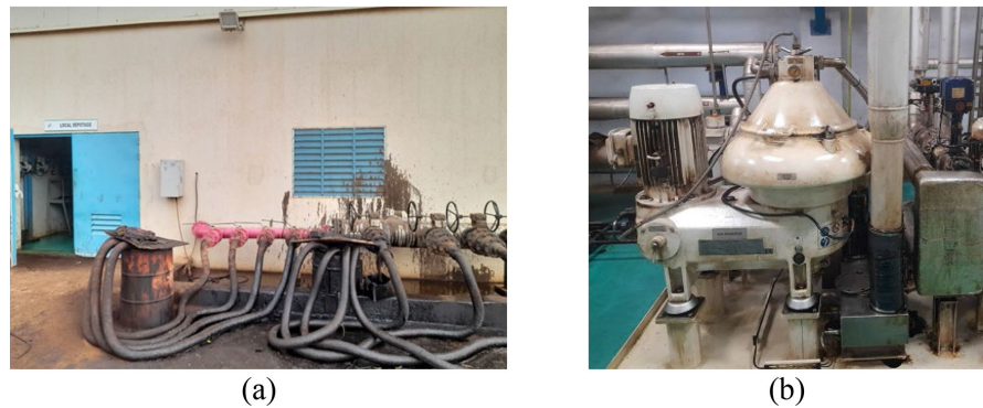
Figure 2. (a) External view of the unloading area at the Ouaga East thermal power plant; (b) HFO separator of the Ouaga East thermal power plant.
