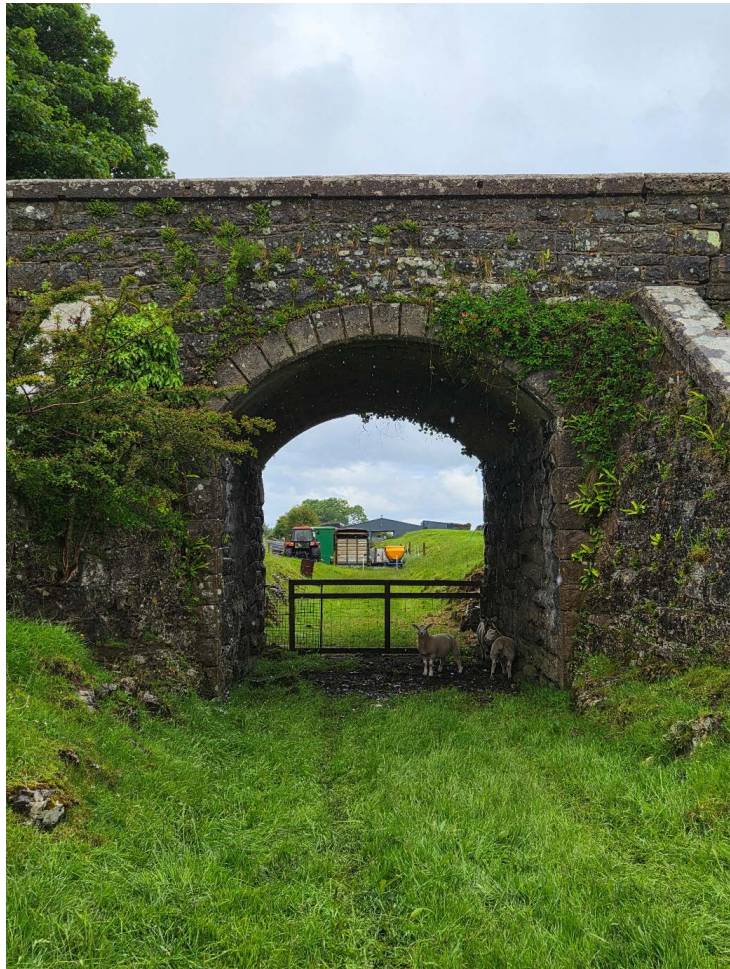
Figure 12. Abandoned CDR Bridge on Public Road (08/06/2026) [23].
