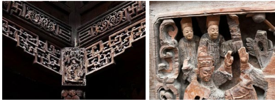
Figure 3. Reinforcing carved brackets and a detailed fragment of wood carving.
